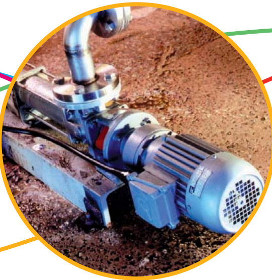
Transfer of industrial detergents
