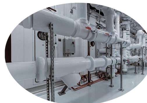
Air Conditioning System
